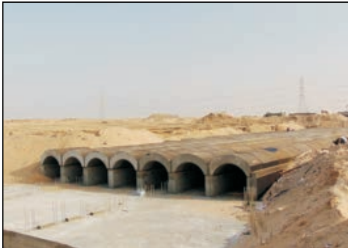
DRAINAGE ARCH CULVERT IN DOWNSTREAM INDUSTRIAL AREA RAS AL-KHAIR REGION, JUBAIL, SAUDI ARABIA
